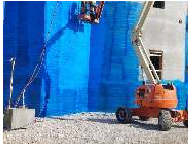
Project: 10,000 SF Slip-Poured Concrete Silo Below-Grade Coated with Ames Blue Max Liquid Rubber Waterproof Membrane.
